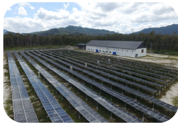
403.2kWp AC coupled 483.84kWp DC coupled
