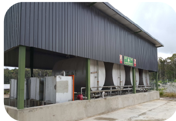
Skid tanks x 4
