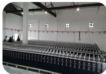
Batteries 3 x 2150 Ah @ 480V
