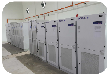
Battery Inverter 600 kW
