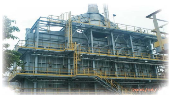
氯乙烯(VCM)裂解爐
