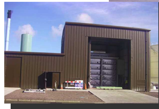
SSE: Shetland NaS Battery 1MW, 6MWhr
