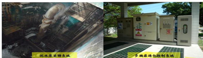
Wastewater Treatment Plant Power Equipment Monitoring and Energy Conservation Management System
